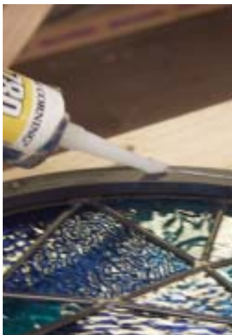
After the desiccant was added to absorb any ambient moisture, then the unit was sealed air and water tight with silicone and then screwed shut. To date, we've had no fogging!
